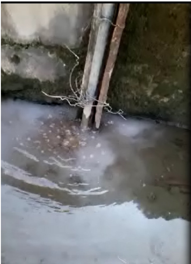
Figure 2: Leakage in main line of water distribution in Sankheda village.
