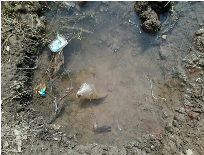
Figure 1: Leakage in main line of water distribution in Sankheda village.
