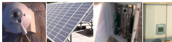
Figure 5: (a) Pyranometer (b) Photovoltaic Modules (c) String connectors (d) Inverter.
